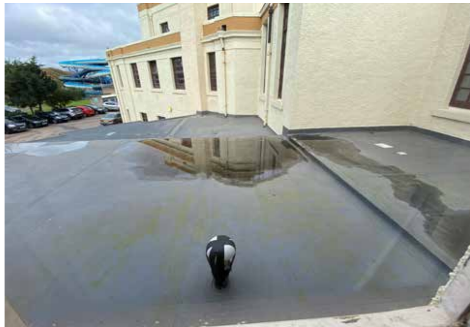
Ponding on L1 roof (left)
